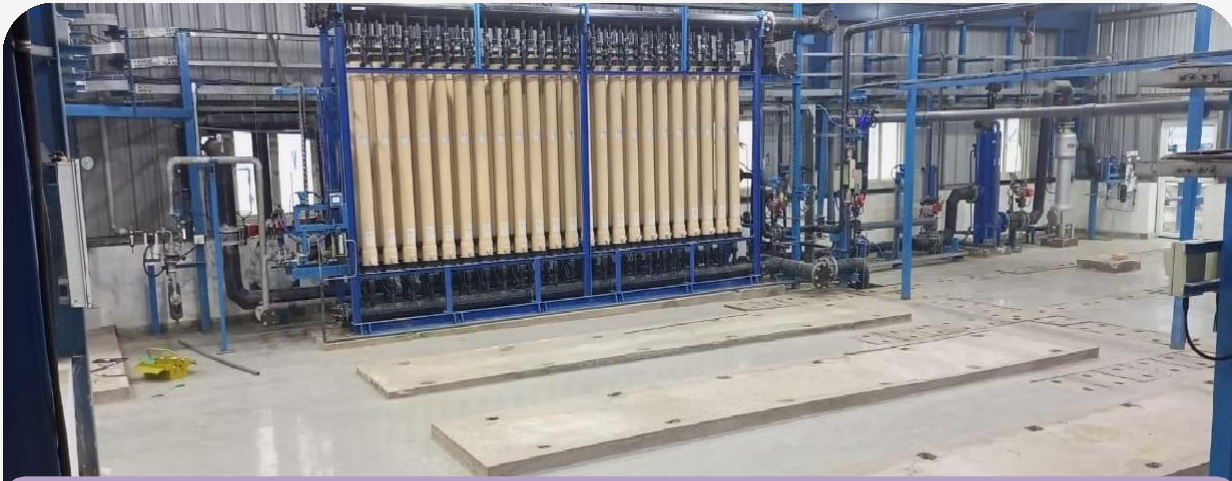
1st Module of UF based 3.125 MLD unit. Membrane for treatment unit procured from Asahi KASEI -Japan
