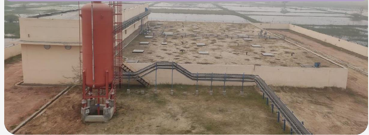
Clear water reservoir of 5 million liters capacity to store treated water
